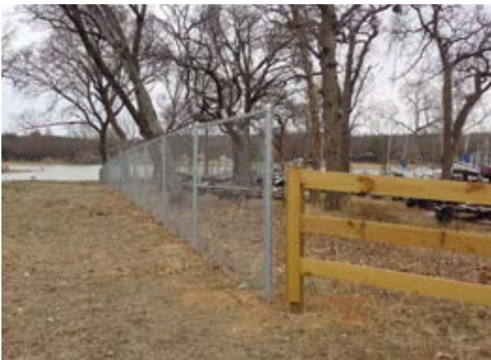
New chain link fence will help keep boats and boat trailers secure.
